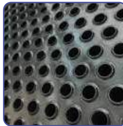
Boilers and heat exchangers
